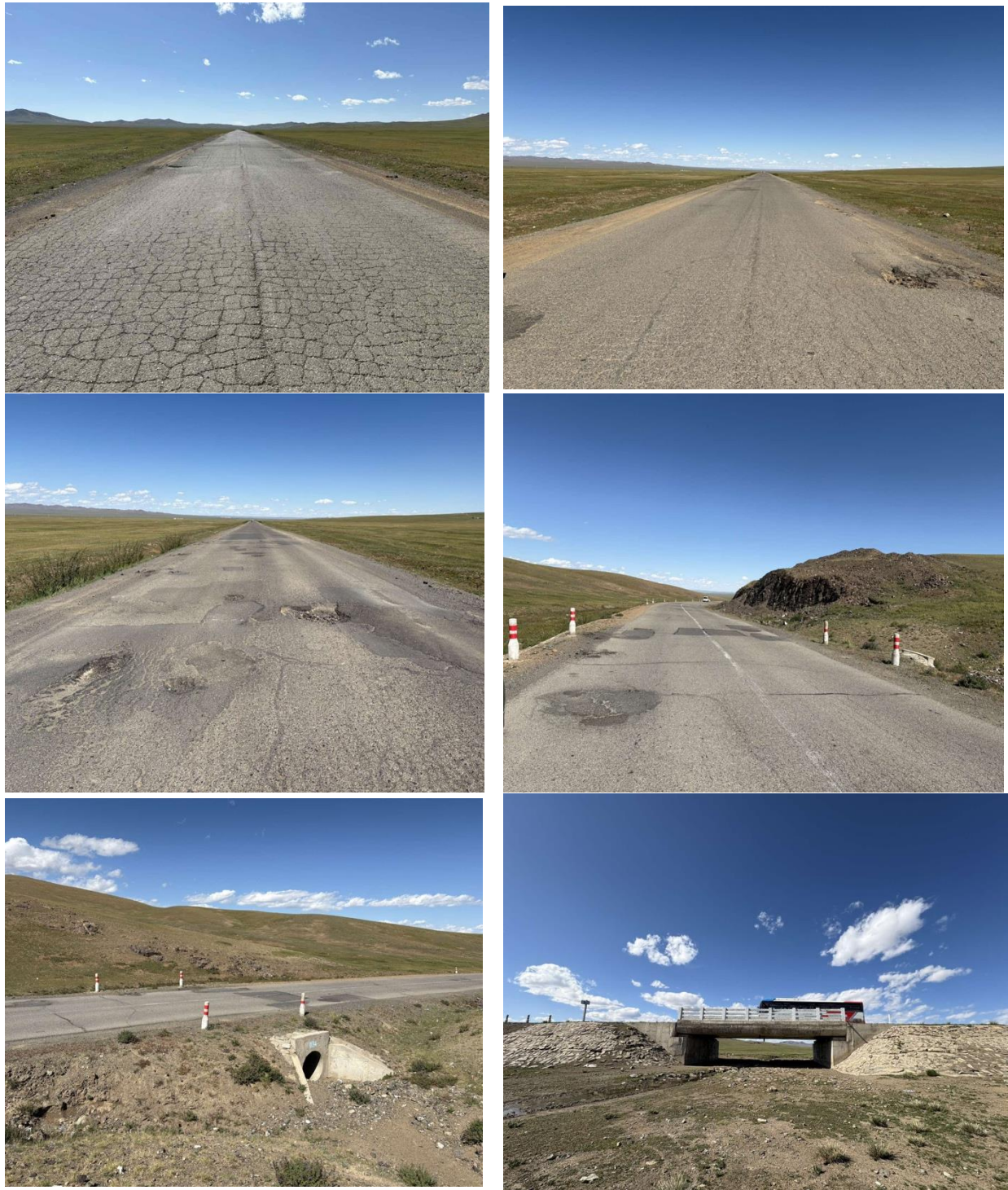
Figure 4. Existing condition of the A0302 road
